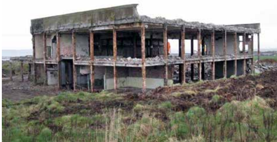
Demolition of the Black Building is underway in November 2009. Photo Steven Heddle
